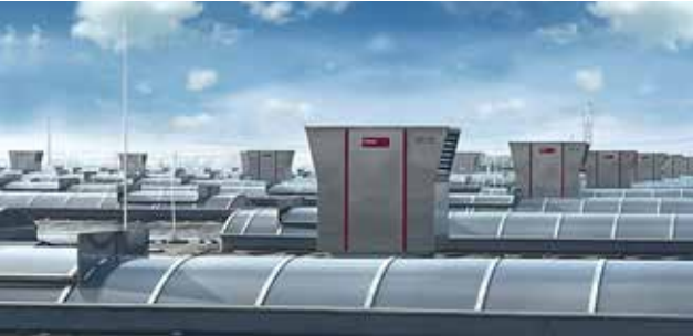
GKN, Miskolc - 28 db Hoval RoofVent® RC, 3 db Hoval UltraGas® 2
