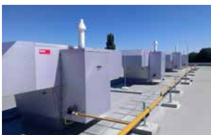
Schott Hungary Kft., Lukácshá- za - 10 db Hoval TopVent®, 4 db Hoval RoofVent® condens
