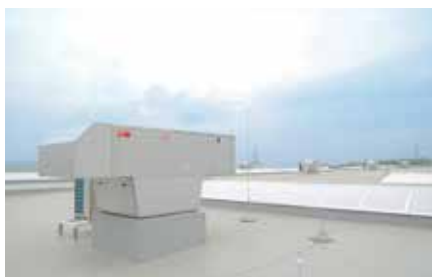
KNAPP Hungary Kft., Nemes- vámos - 13 db Hoval RoofVent® twin pump LW
