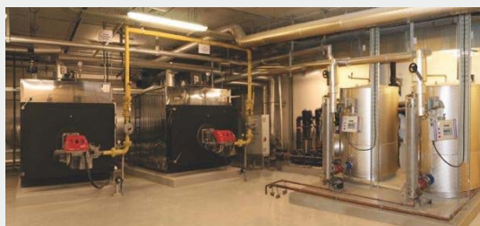
Al Meydan Racecourse, Dubai ECOTHERM Turnkey Hot Water & Steam System
